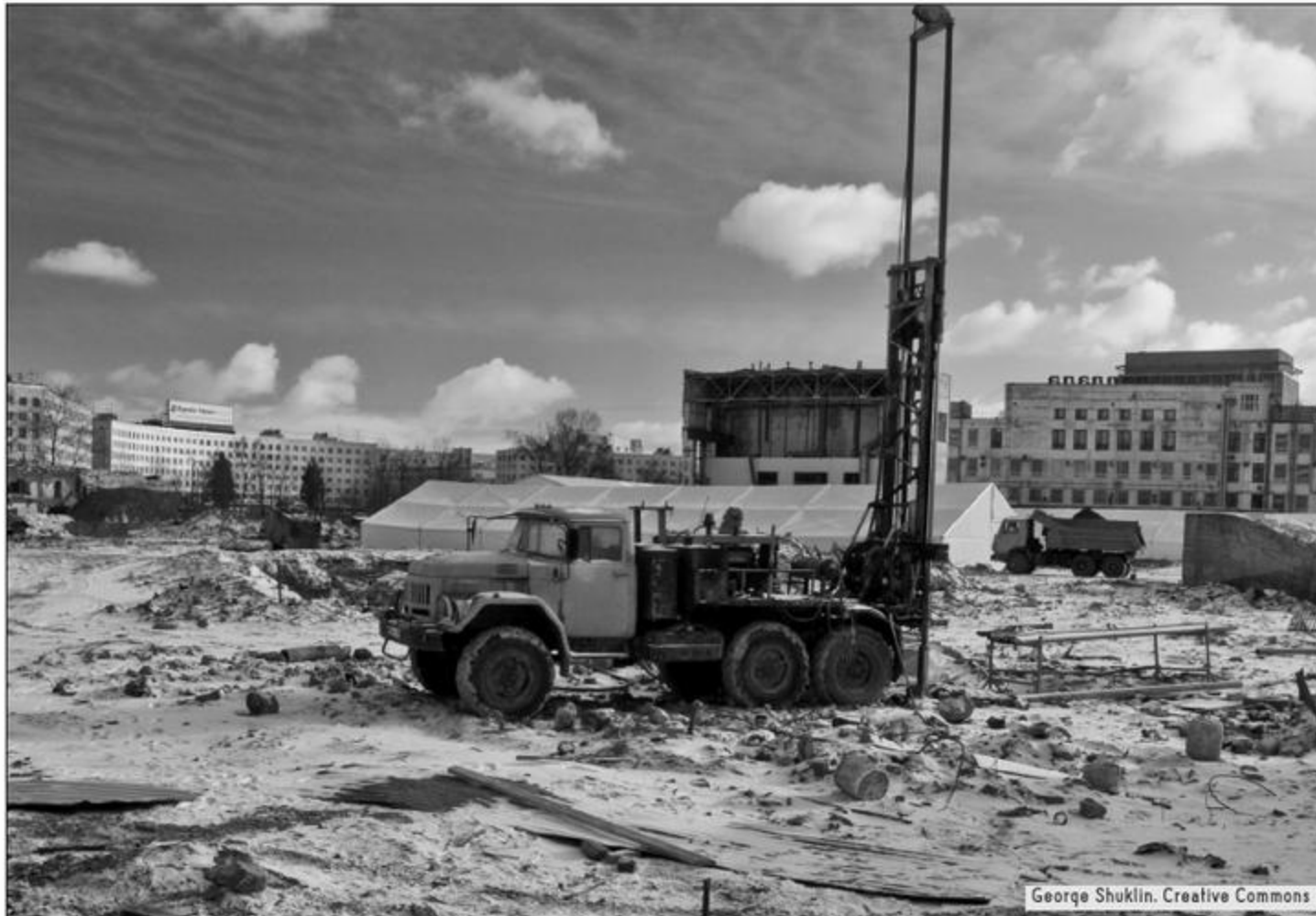
Okhta Center, a skyscraper being built by Russian oil and gas monopoly Gazprom, under construction in 2008. The ability to build huge projects like this one demonstrates Gazprom's immense wealth and power.
